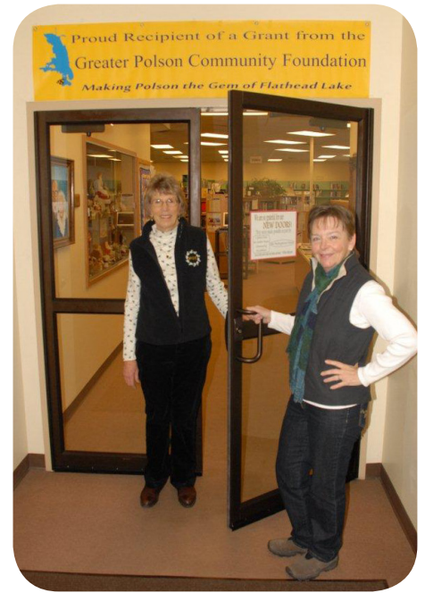
Penny Jarecki (left), President of the Greater Polson Community Foundation (GPCF), and Jackie Gran, Chairperson of the Board of Trustees for the North Lake County Public Library District, swing open new doors recently installed at the library. Two sets of glass doors, partially paid for with a grant from GPCF, are the first of several renovations planned for the library.
